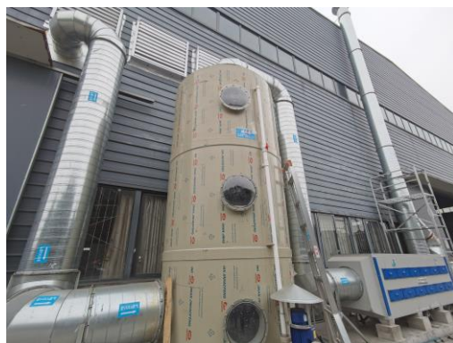
喷淋塔+两级活性炭+16.5m 排气筒 DA003
