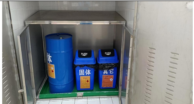
危废暂存点防渗托盘
